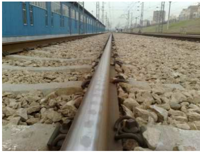
Figure 12. Rail corrugation at the tangent track
