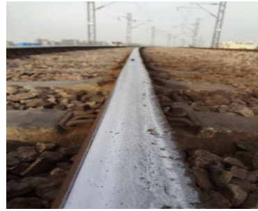
Figure 13. Rail corrugation at the curve
